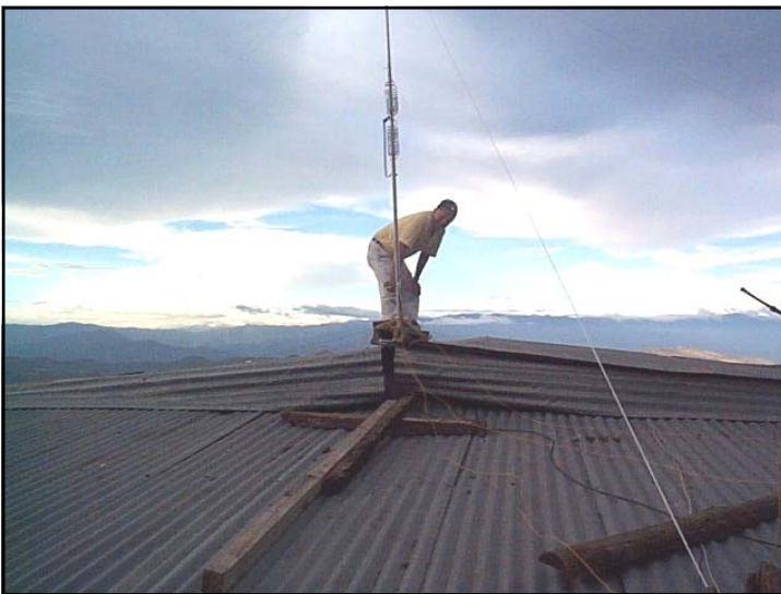
That's me, carefully inspecting the Butternut HF-2V installation.
