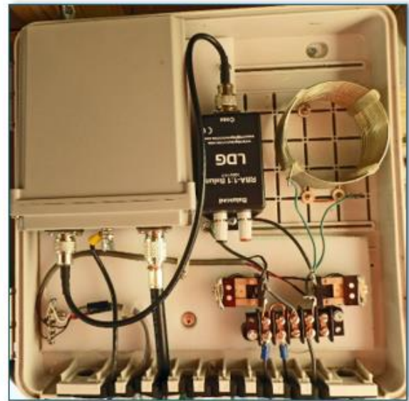
Figure 3. Low band remote auto tuner, balun, and 80-meter loading coil.
